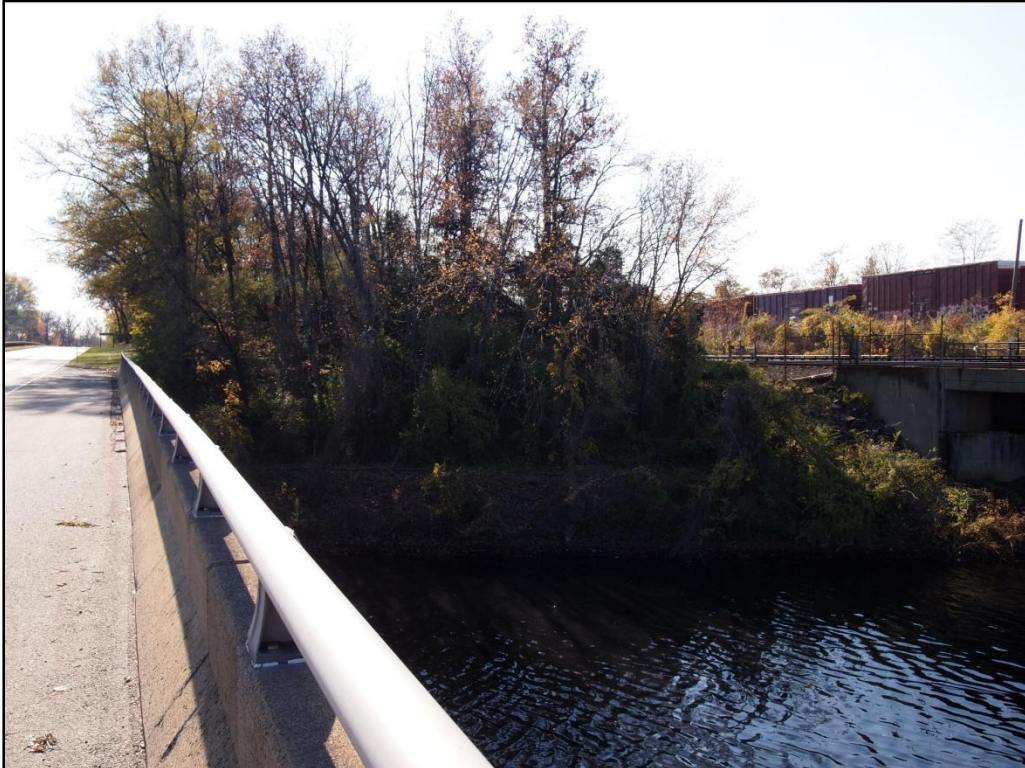
Plate 11: View southwest of the southbound side of the MVMH/PNCR south of Four Mile Run showing area where vegetation would be removed as part of construction of the proposed Build Alternative D.
