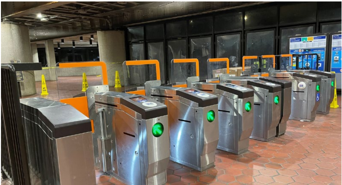
Faregates at station
