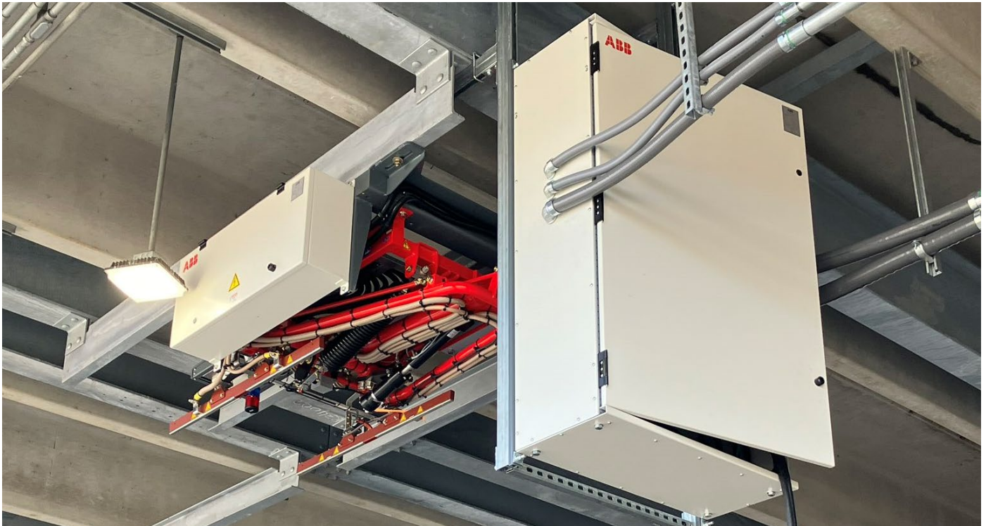
Zero-emission electric Metrobus Pantograph charging station FY2025 funding constraints could impact future investment in the Zero-Emission Bus Program
