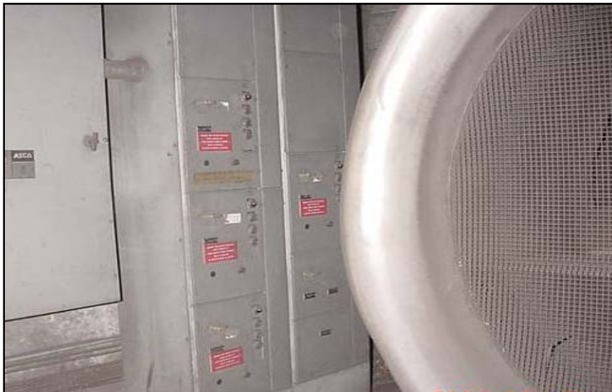
Serves Ventilation Fans & Drainage Pumps
