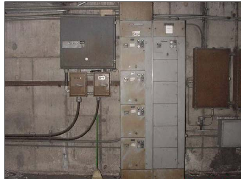
Motor Control Center
