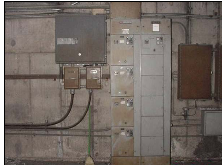
Motor Control Center
