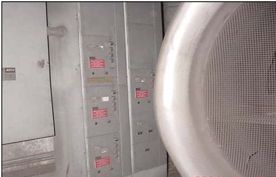
Serves Ventilation Fans & Drainage Pumps
