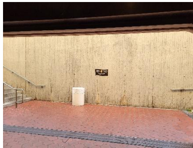
Figure 2: Riders exiting the station to the west are greeted by an uninviting concrete wall that blocks all visibility of the surrounding areas.
